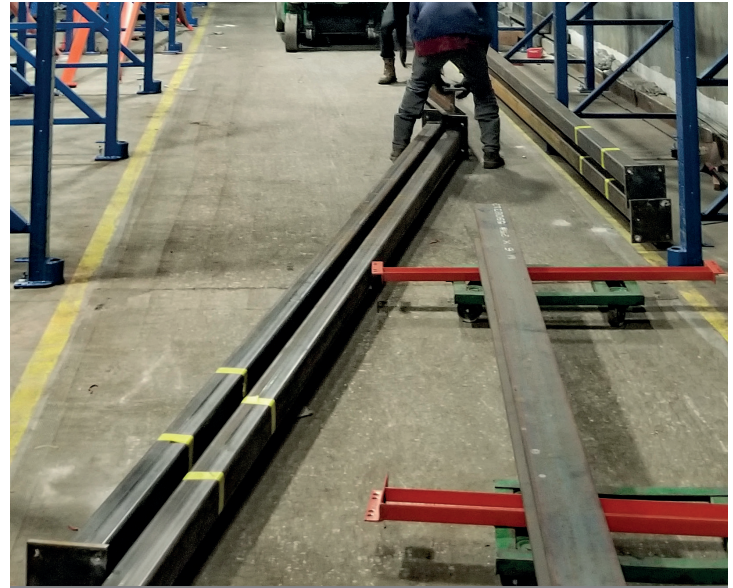
Temporary columns support ceiling while rack is dismantled & replaced row by row.
